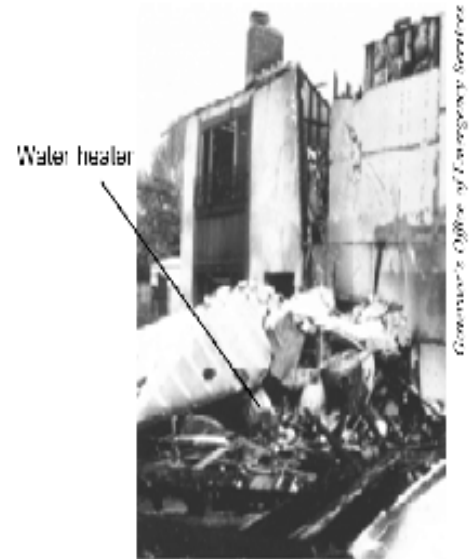
Figure 10 - The unbraced water heater in this building fell during an earthquake; the resulting fire destroyed the building.
