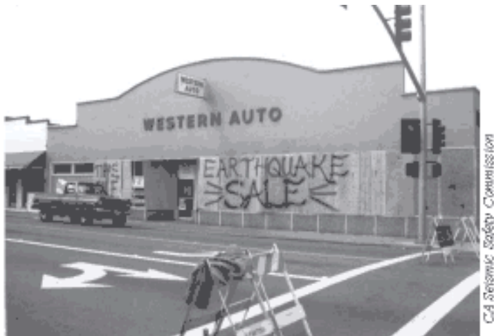
Figure 55 —The front window of this Fortuna auto parts store broke in the 1992 Cape Mendocino earthquake.
