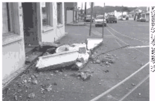
Figure 20 - Unbraced Parapets can Injure and Kill - This parapet on the front of the building in Figure 18 fell on the sidewalk.
