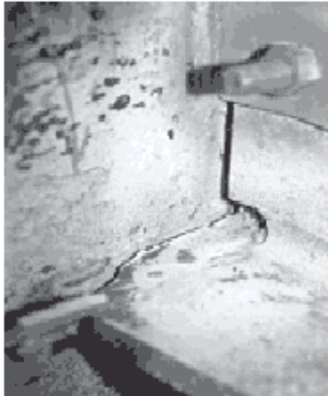
Figure 27 —This steel frame connection unexpectedly cracked in the 1994 Northridge earthquake.
