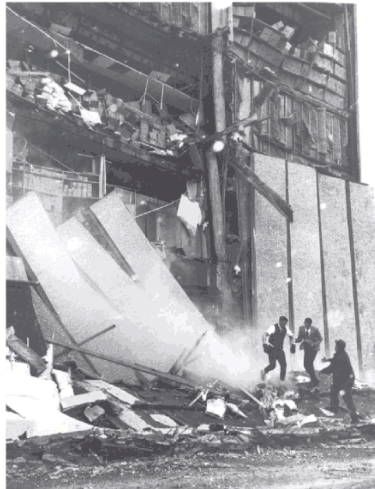
Figure 37 - Cladding on this store in Anchorage failed in the 1964 Alaska earthquake.
