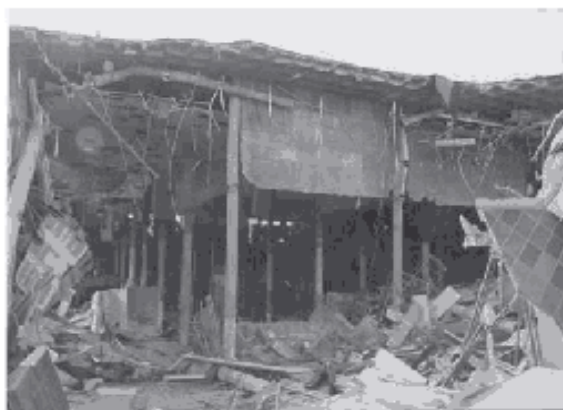
Figure 4 - Department Store Collapse in Northridge 1994. Fortunately no lives were lost since the earthquake occurred before store hours.
