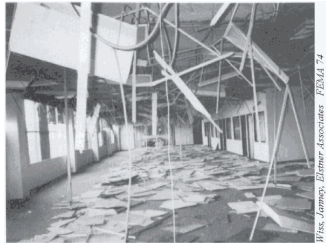
Figure 53 - This building sustained extensive interior nonstructural damage during the 1994 Northridge earthquake. Parts of the ceiling grid and tiles have fallen.
