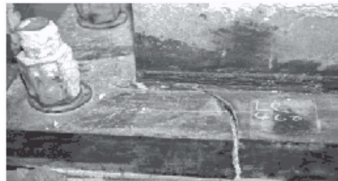
Figure 28 —A 4-inch-thick steel plate supporting the base of a column at the Oviatt Library at CSU Northridge fractured in the 1994 earthquake.
