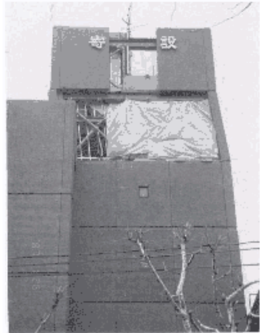
Figure 29 —A six-story steel braced frame building was damaged after the 1995 Kobe Earthquake in Japan. 4,000 to 8,000 small commercial buildings and 1,000 to 2,000 large commercial buildings were destroyed or severely damaged in that event.
