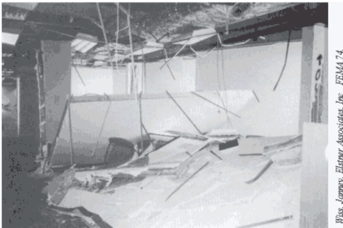
Figure 60 - Partitions and ceilings toppled onto office spaces during the 1994 Northridge Earthquake.
