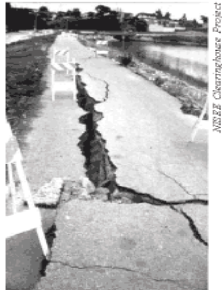
Figure 67 - Lateral Spreading. Loma Prieta Earthquake, October 17, 1989. Lateral spreading damage levee road along the San Lorenzo River.
