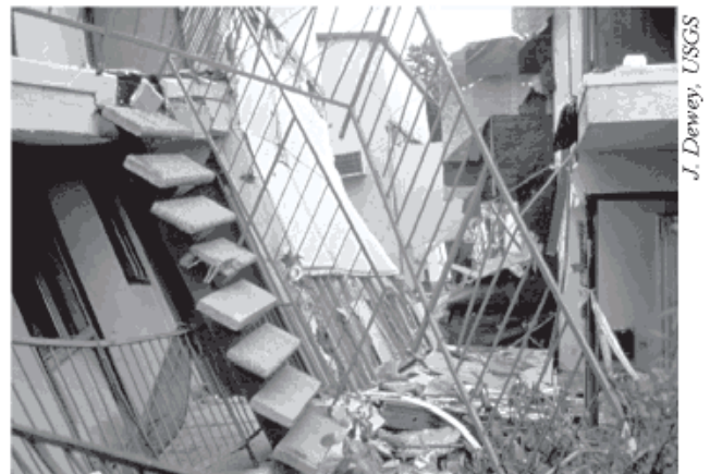
Figure 36 - Stairs to an apartment building collapsed during the 1994 Northridge earthquake.
