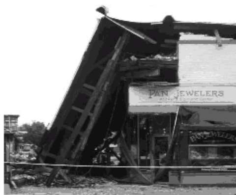
Figure 6 - San Simeon Earthquake, Dec. 22, 2003. The Acorn Clock Tower Building constructed of unreinforced masonry collapsed killing two people.
