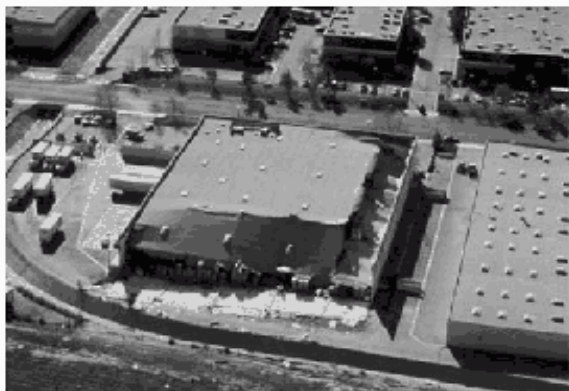
Figure 1 - Partial Collapse of an Industrial Building. Poor connections between the walls and the roof caused this collapse.
