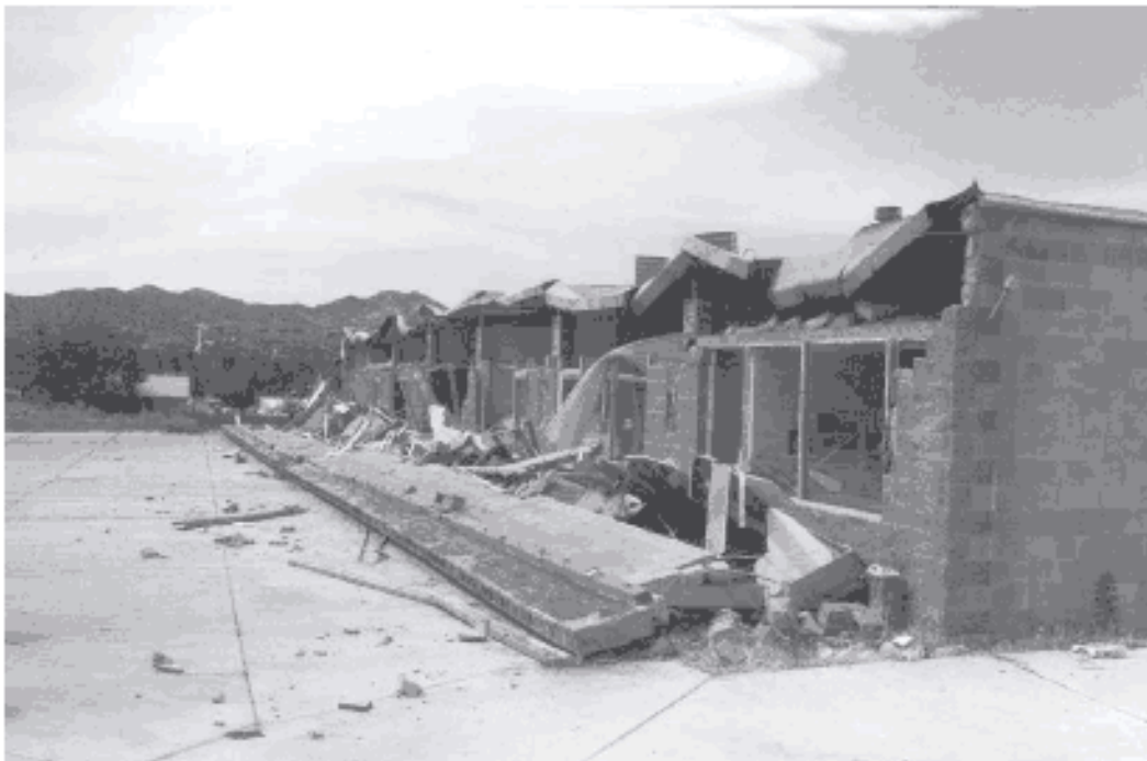
Figure 15 — Wall Anchors Can Prevent Failures Like This. Even newer buildings are not immune to earthquakes. This reinforced masonry strip mall was built in the 1980's but did not comply with the building code. The wall anchorage failed in the 1992 Landers Earthquake. Its front wall fell into the parking lot.
