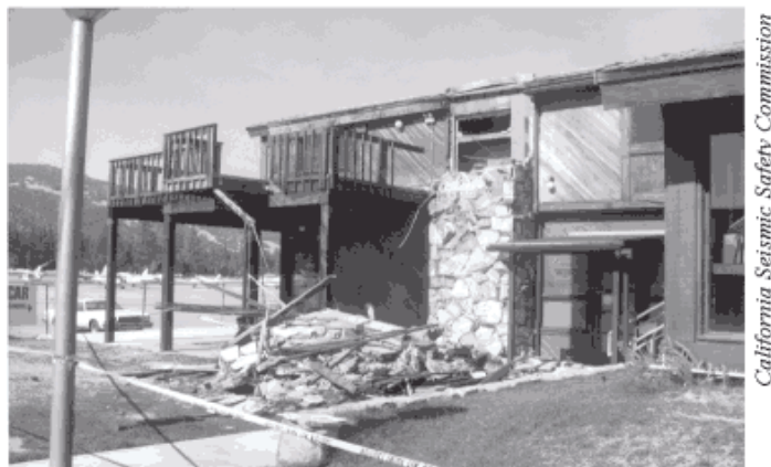
Figure 35 - The chimney on this building fell on the stair-way in the 1992 Big Bear earthquake, cutting off a means of escape for persons on the second floor.
