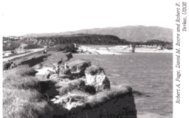
Figure 69 - Lower San Fernando Dam that was badly damaged by the 1971 San Fernando Earthquake.
