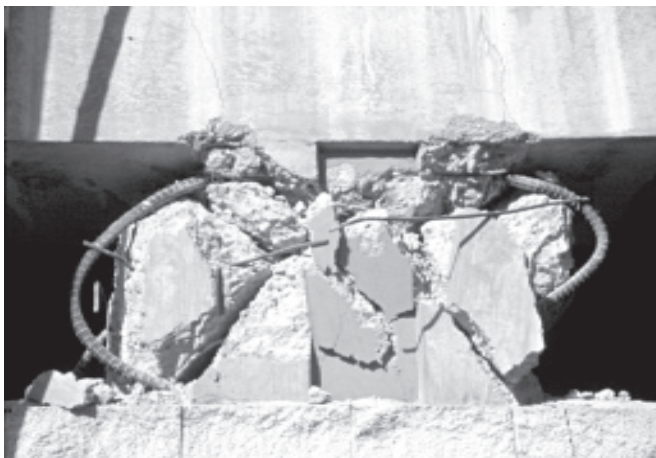
Figure 22 - Short columns in this parking structure failed in the 1994 Northridge earthquake. Modern building codes now require much more reinforcing steel for such short columns.
