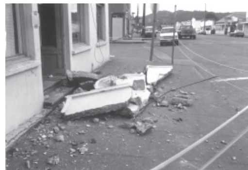
Figure 20 - Unbraced Parapets can Injure and Kill - This parapet on the front of the building in Figure 18 fell on the sidewalk.
