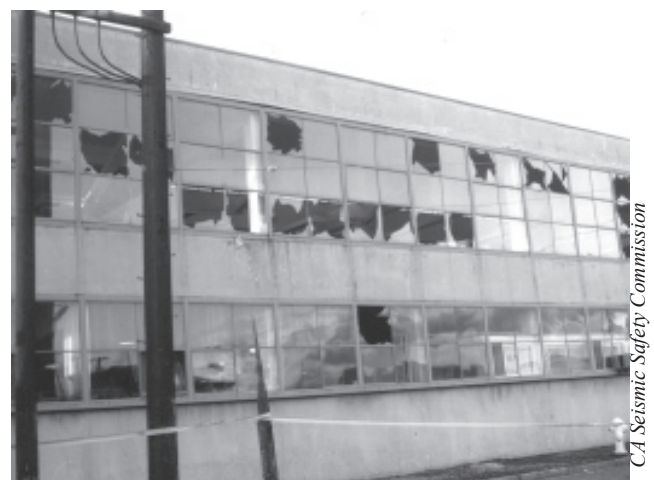
Figure 56 —The windows in this San Francisco building probably broke because its frame flexed too much in the Loma Prieta earthquake of 1989.
